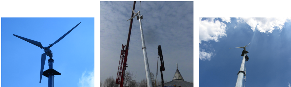
Figure 5.22: Rotor of the HY5kW wind turbine (left), lifting of the turbine for installation (middle) and low-tech procedure to level the turbine (right).
